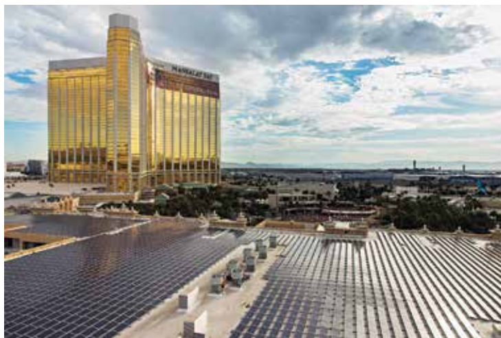
This solar array, one of the largest in the world, takes up nearly 20 acres of roof space atop the Mandalay Bay Convention Center.
